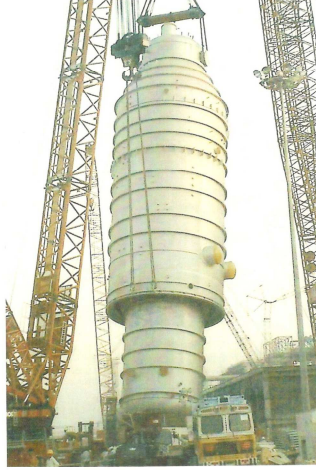
UNIT : CRUDE, RIL SEZ EQUIPMENT : VACCUM COLUMN WEIGHT : 550 MT
